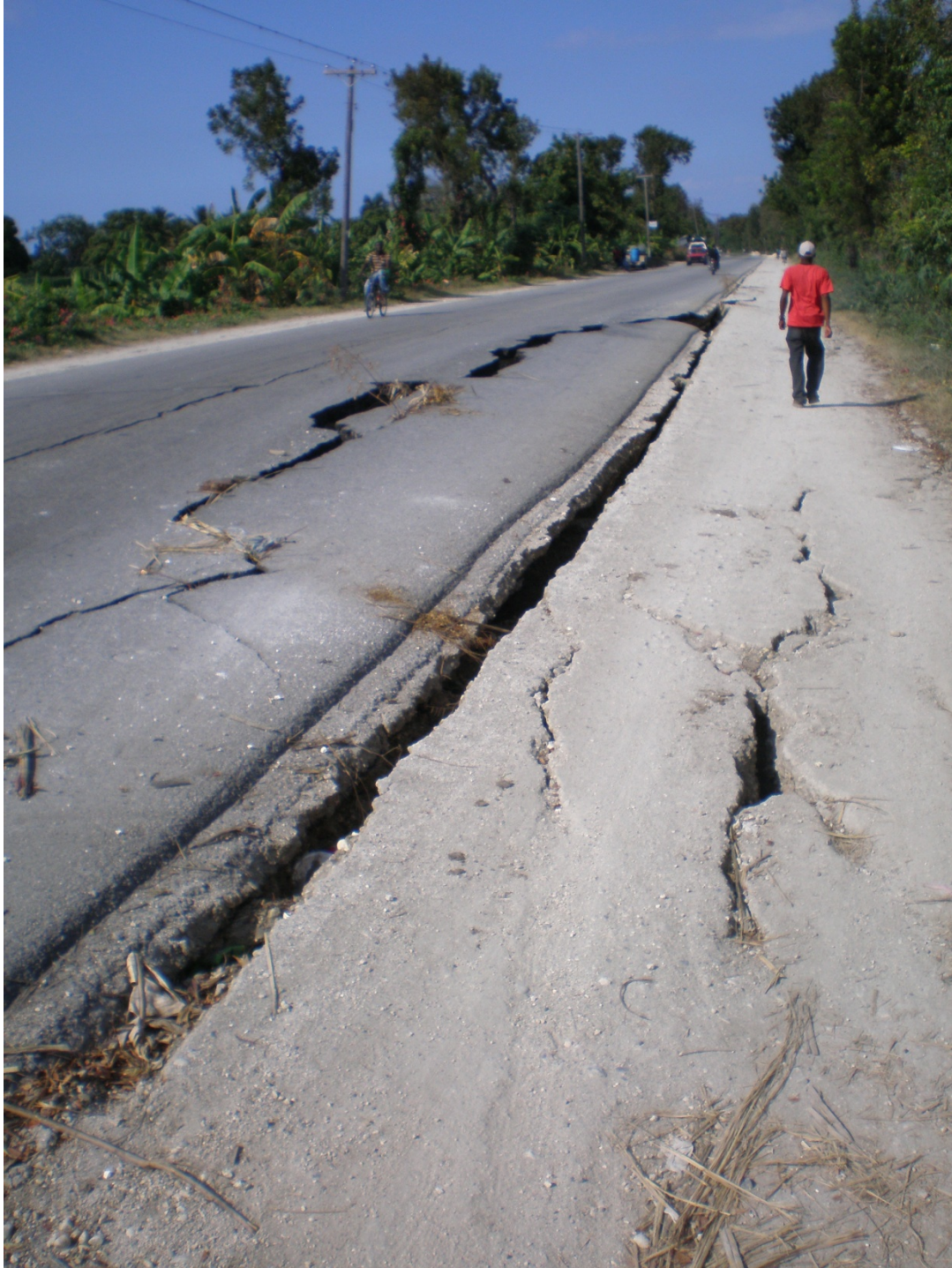
Figure 8.5 Cracks induced by fill slope slumping at road damage site BOXCLVTA.
