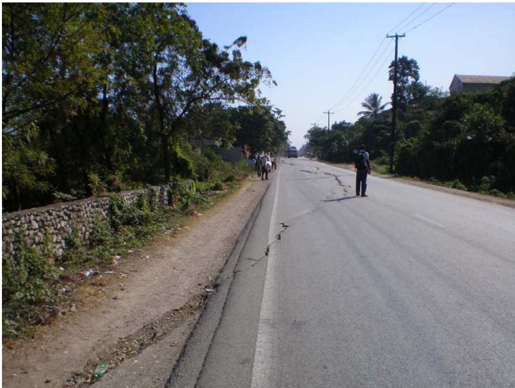
Figure 8.4 Typical arcuate road cracks at road failure site RCA west of Carrefour.
